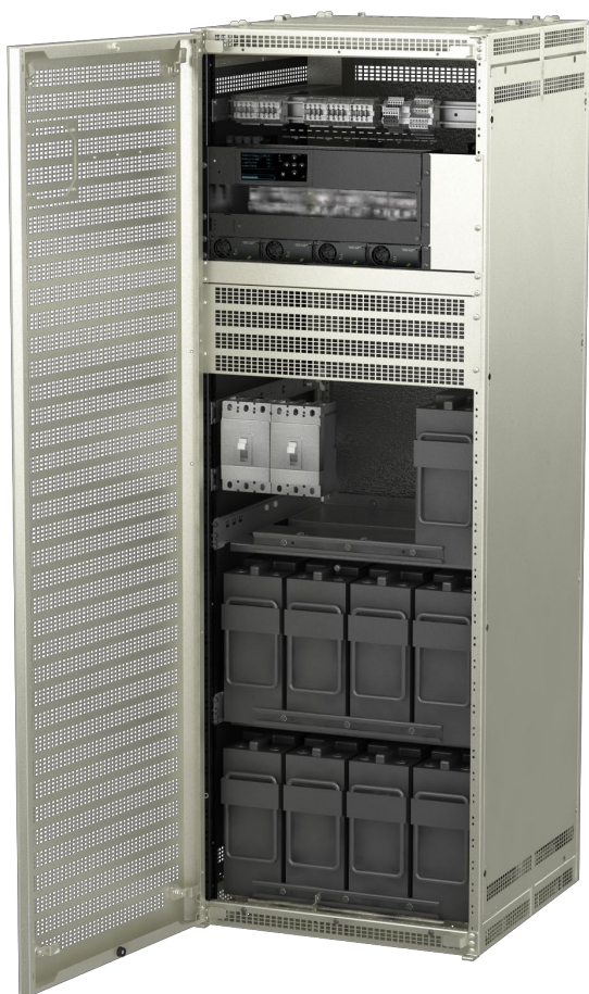
IBB system in FPC cabinet
