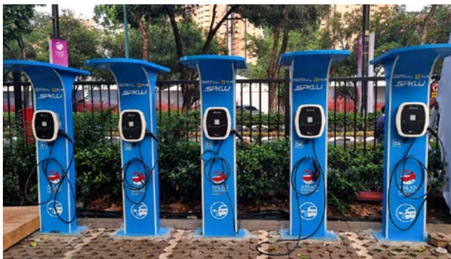
Delta set up a total of 80 charging facilities in Jakarta, Indonesia for the 43 rd ASEAN Summit
