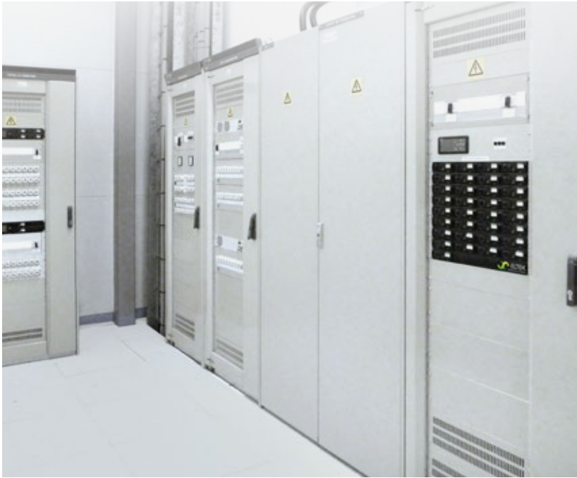
Complete AC and DC systems with distribution
