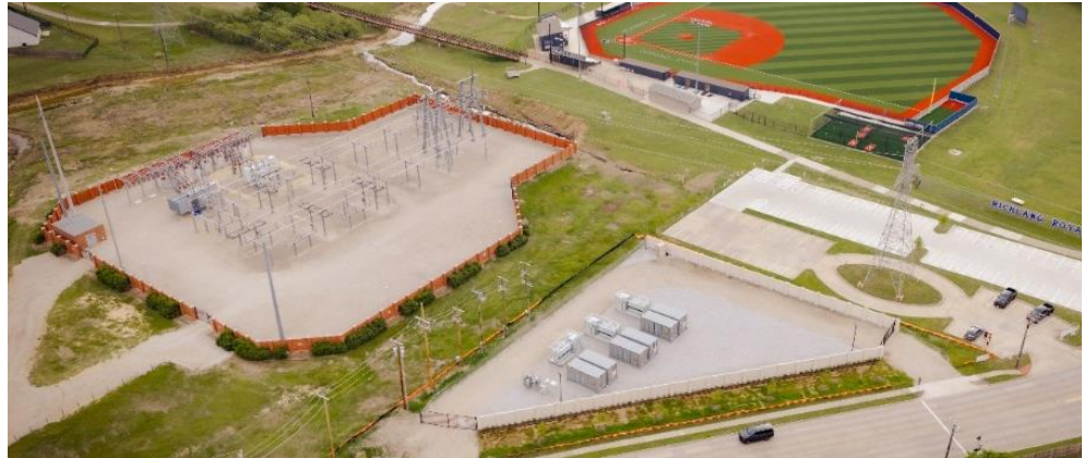
Meadow Park, a 12.9 MW battery energy storage system outside Plano, Texas.
