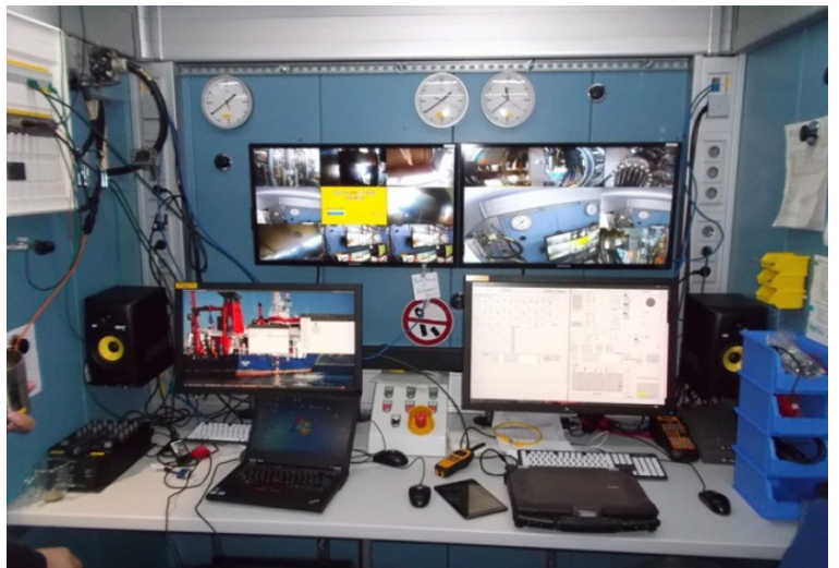
• Delta's DVCS enables the operators in control room to manage the MEBO drilling
