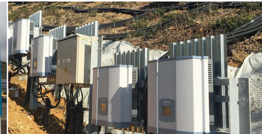
The Park uses 185 units of Delta's RPI-M series PV inverters which feature strong enclosure to withstand adverse weather conditions.
