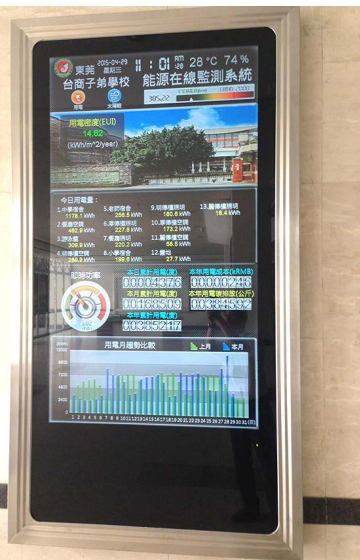
The Delta Energy Online system is used to monitor energy use throughout the entire campus of a local elementary school for children of overseas Taiwanese. it.
