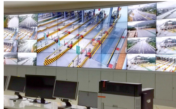
Shenzhen–Luoding Expressway uses Delta large screen display system for traffic management.
