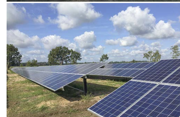
Delta turned an abandoned building into 1.56MW PV plant featuring M50A inverters.
